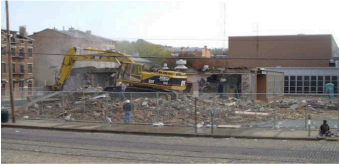
Note. A student of Washington Park Elementary School Looks on as Demolition Begins.
